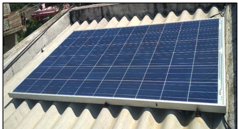
Solar panels installed on the roofs of Single Teacher Schools to provide electricity for evening classes
